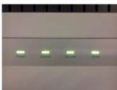
System Status Lights
